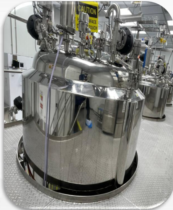
MIXING & PRESSURE TANKS
