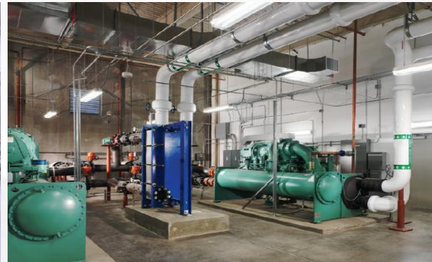
UTILITY PIPING SYSTEM
